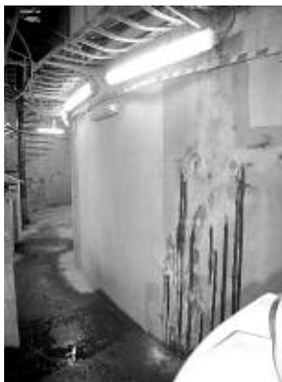
Rysy i zacieki na ścianie zbiornika Cracks and stains on the wall of the tank
