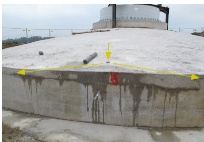
Photo 4. Water flow along the delamination in concreting/„cold joint” at a considerable distance from the place where the control drilling was made on the upper surface of the foundation
