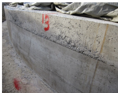
Photo 2. Horizontal break in concreting („cold joint”) and an under-compacted layer of concrete („honeycombing”) – the side surface of the foundation
