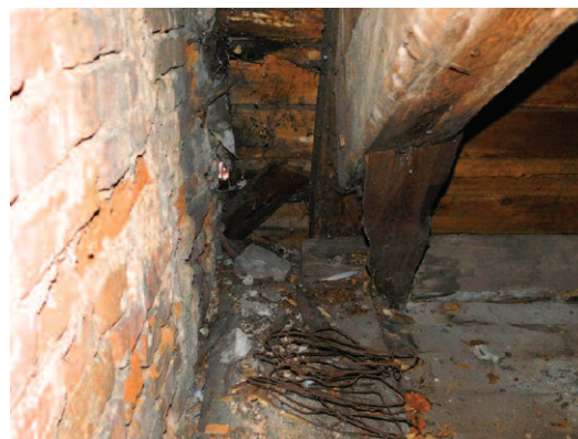
Photo 5. Damage of the wall-side rafter caused by fungi
