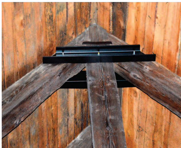
Photo 8. Implementation of the strengthening of the joint between the rafter and the king post at the ridge
