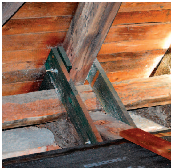
Photo 7. Implementation of the strengthening of the joint connecting the rafter and the beam
