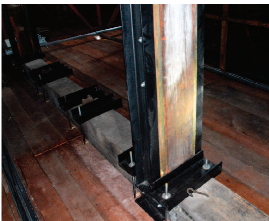
Photo 9. Implementation of the strengthening of the joint between the king post and the main beam
