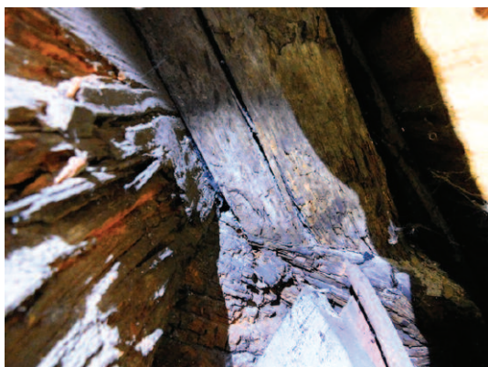
Photo 4. Prismatic cracking at the joints between rafters bottom purlins and tie beams
