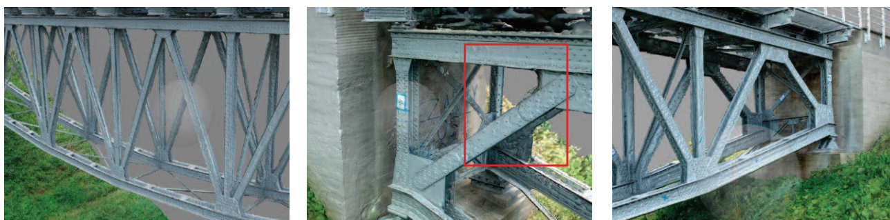
Photo 2. Segments of the truss in global model, with the portion corresponding to the local model highlighted in red
