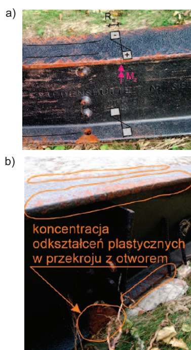
Photo 3. Interpretation of the state of deformation in the beam around section B – description in article
