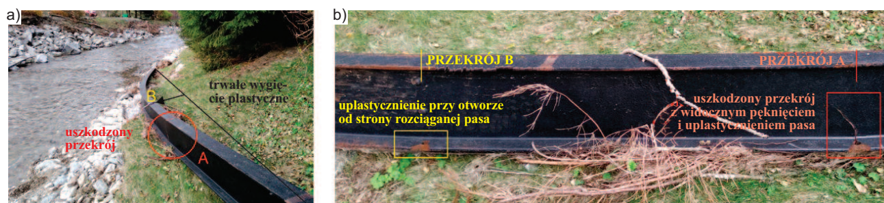
Photo 2. I320 steel beam with holes in the lower chord found below the bridge
