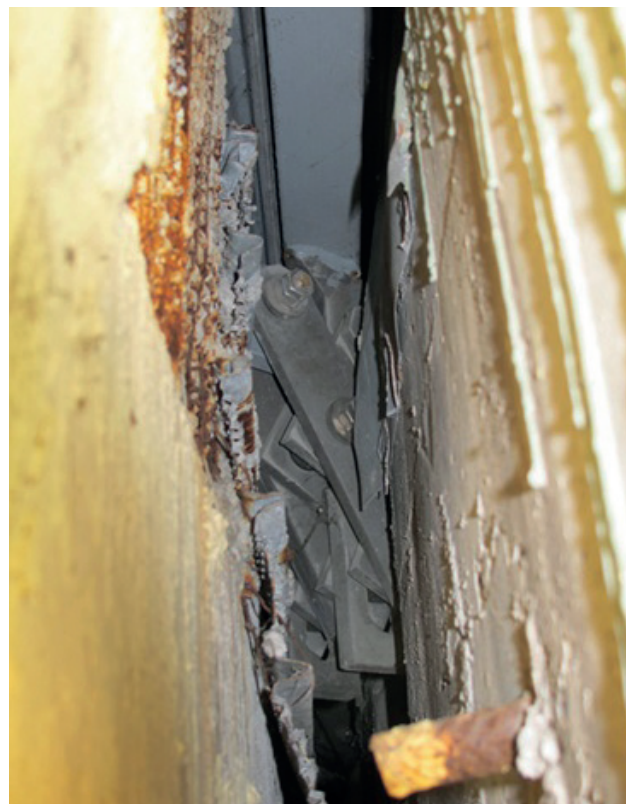
Photo 3. Two-module expansion joint installed in an expansion joint gap of insufficient width and in niches that are too small
