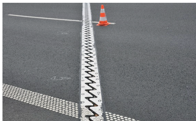
Photo 1. View of the nosing expansion joint with noise reduction plates with the pavement made too low
