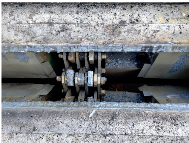
Photo 6. Incorrect positioning of the modular expansion joint in the plan
