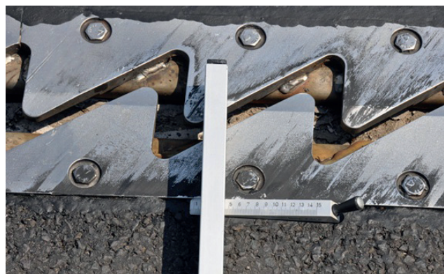
Photo 2. Height difference of 4.5 mm between the pavement and the upper surface of the noise reduction plates
