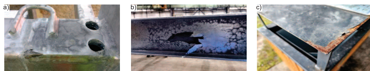
Photo 2. Consequences of the use of wrong type of steel: a) dull HDG coating with cracks and local delamination; b) brittle HDG coatings with poor adhesion to the steel; c) dull, brittle coatings with poor adhesion to the steel
