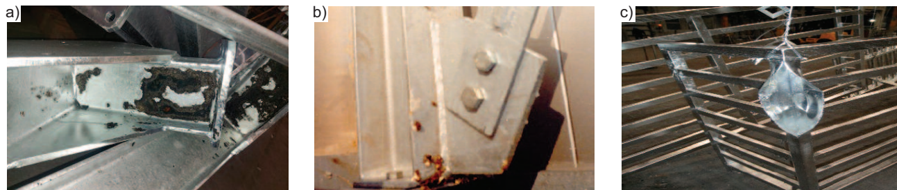
Photo 3. Effects of incorrect steel surface preparation before galvanizing: a) surface preparation defects and lack of technological holes; b) leaking corrosion products; c) view of a torn element after an explosion – lack of a hole for venting the structure
