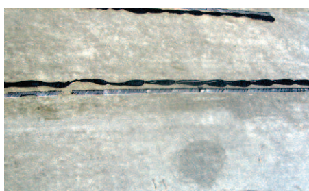
Photo 3. Discolorations on the removed fibre-cement cladding, which may indicate decreased strength properties
