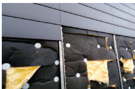
Photo 2. Expanded mineral wool with damaged wind barrier
