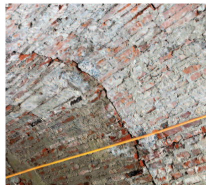
Fot. 7. Spękanie sklepienia garażu [4] Photo 7. Cracks in the garage vault [4]
