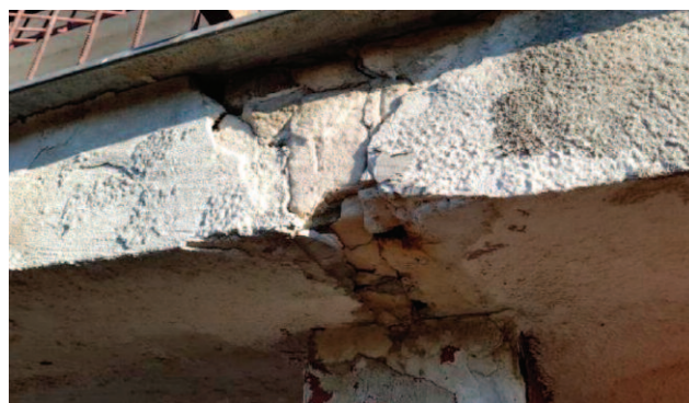
Lublin 2020. Ubytki w złączu prefabrykatów loggii [2] Lublin 2020. Defects in the joint of prefabricated loggia [2]
